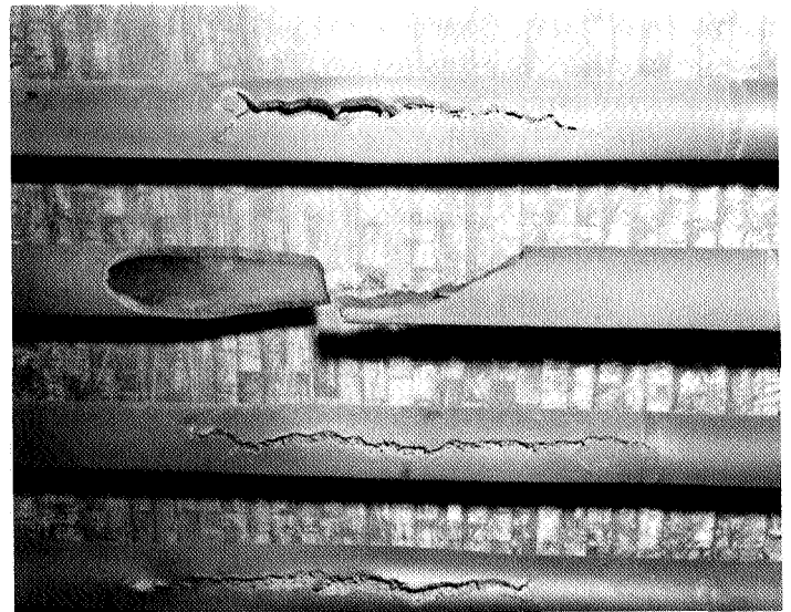
Figure 6. Reformer Tubes Shortly after a Series of Flame-outs
